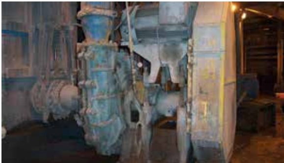
SRL-XT 14×12–36 on Ball Mill Discharge Service
